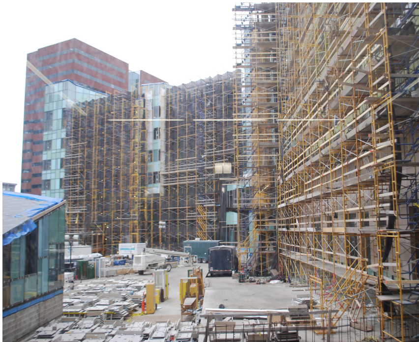
Construction of the new building for the Sloan School of Management at MIT by the firm Moore Ruble Yudell.
